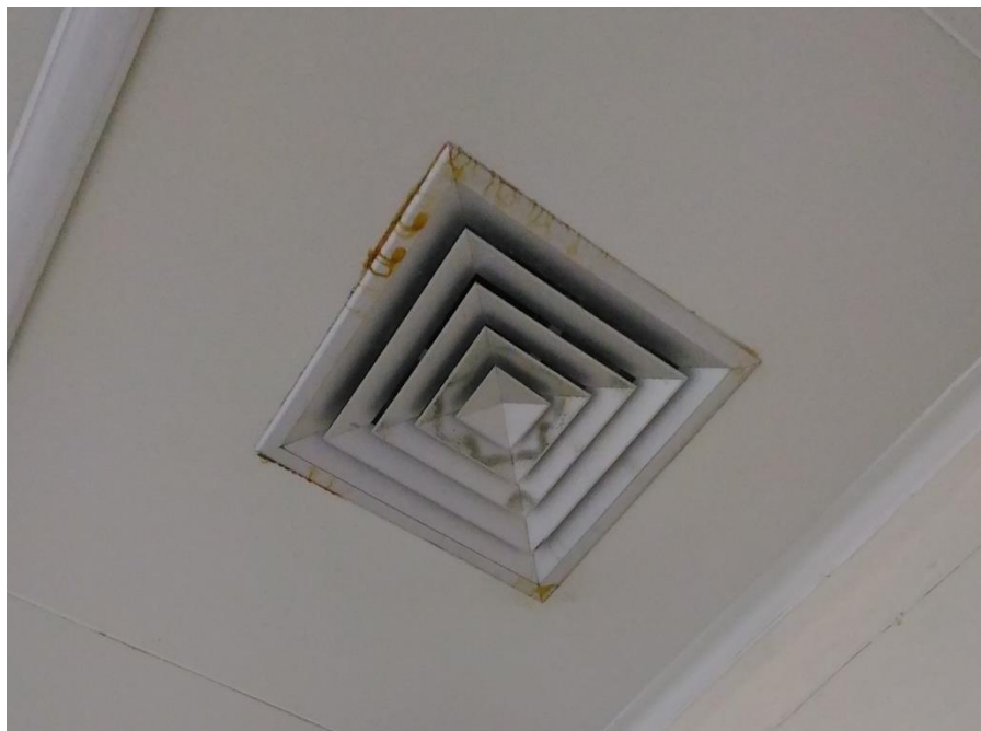
Exhaust Fan di ruang operasi
