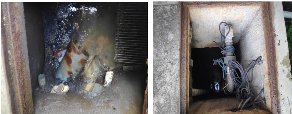
Gambar 12 Inlet IPAL/Collecting Tank 1 dan 2
